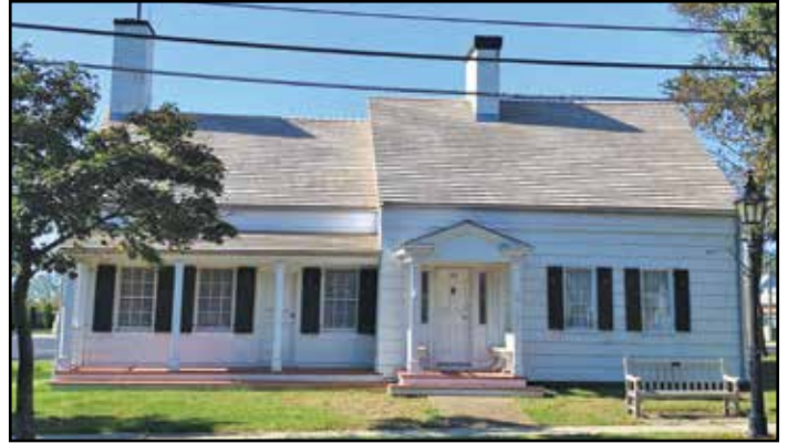
Check out the beautiful new roof and gutters on the Tuthill House!
